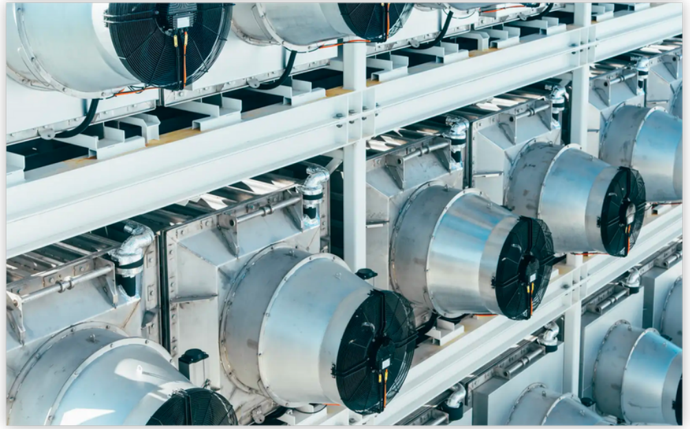
Orca DAC plant in Iceland. Credit: Climeworks
