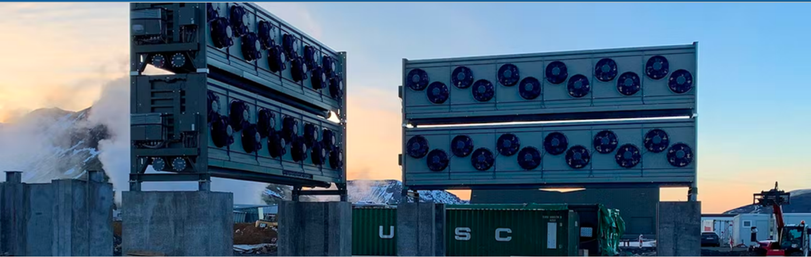
The mounting of the first four collectors at the Orca Direct Air Capture plant, Reykjavik, Iceland. Credit: Climeworks.
